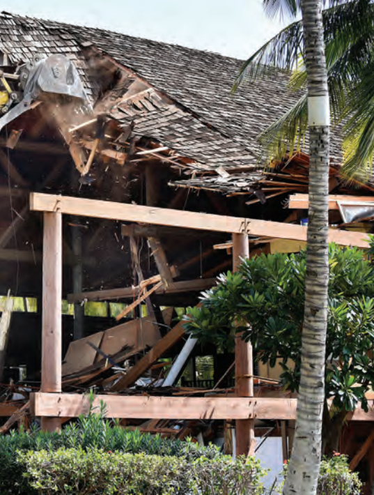
Demolition of former Aston Maui Lu PHOTO COURTESY MATTHEW THAYER, MAUI NEWS
